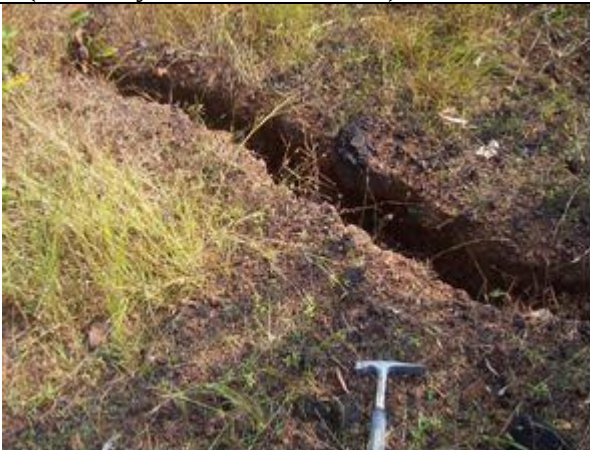
Photo 10: Cracks observed in the mid portion of crown
