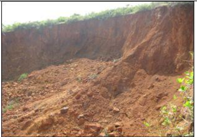
Photo 4: View of top portion of Kadwad landslide
